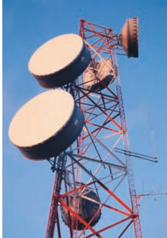
Figure 20 The antenna at the top of a microwave tower receives signals from nearby cell phones. Are any microwave towers located near your school or home? Where?
